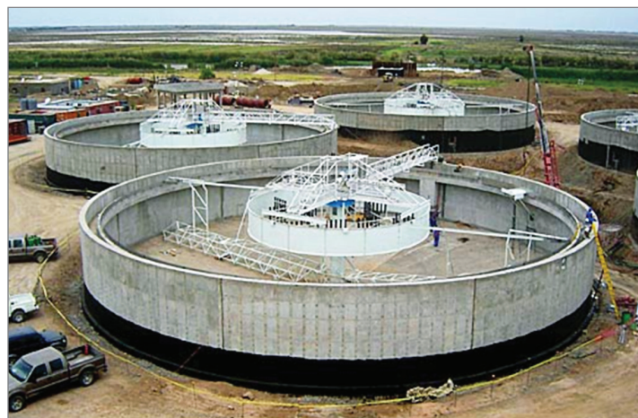
The Nassiriya water-treatment plant, Iraq, 2007. (U.S. Army Corps of Engineers photo)
